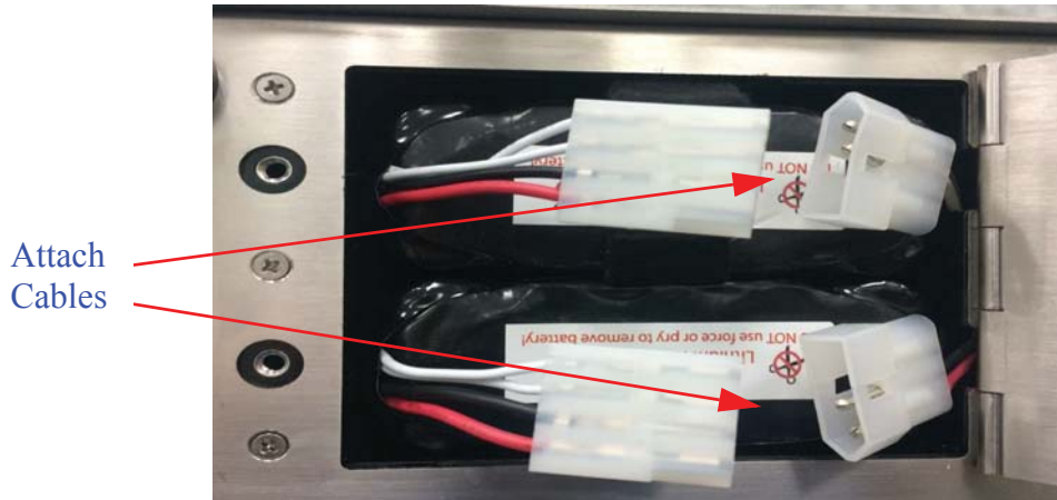
Figure 3-6 Dual-Battery Compartment With Batteries
